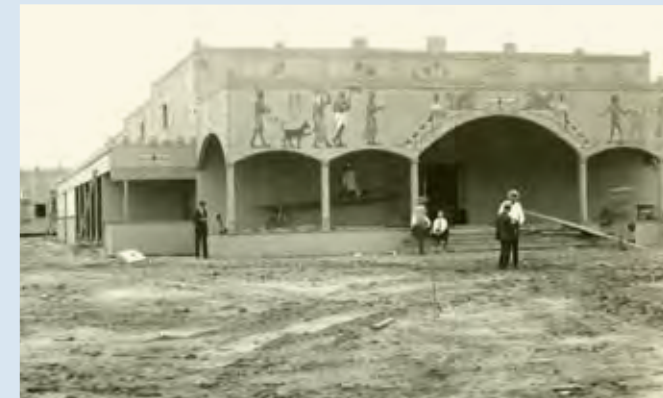
Construction of the Streets of Cairo exhibit, June 1926. This exhibit was part of the "Through the Orient" section of the Exposition, providing visitors a chance to experience the exotic lands of Egypt. This location is the approximate site of the former U.S. Naval Hospital, which today is a surface parking lot, west of the Eagles' NovaCare Complex.
