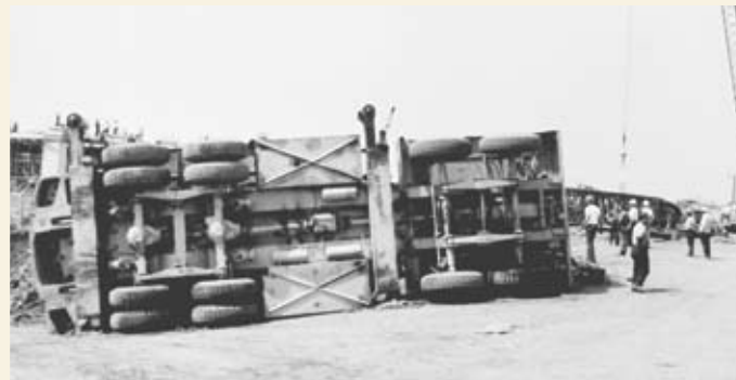
Three workers were injured when a 140-foot crane toppled during stadium construction, May 16, 1969.
