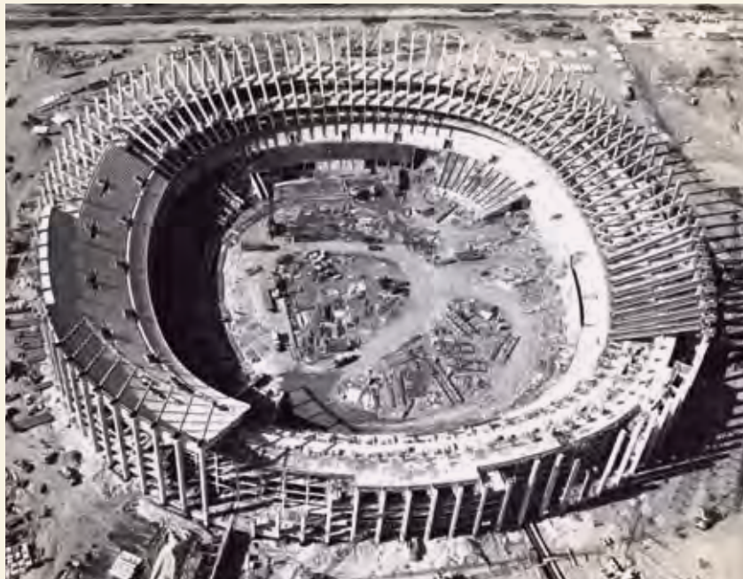
Aerial view of construction, November 2, 1969. The "octorad" design made the stadium compatible for both baseball and football games.
